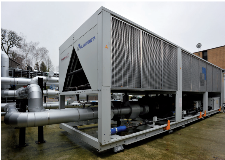
Figure 2 One of ECMWF's Turbocor based chillers.
