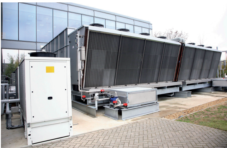
Figure 3 External view of a typical free cooling module. Photograph provided courtesy of Keysource ( www.keysource.co.uk ).
