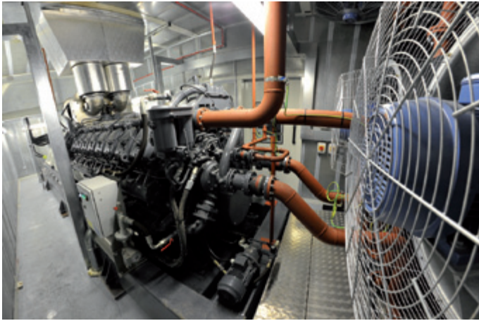
One of ECMWF's high-capacity UPS machines.
